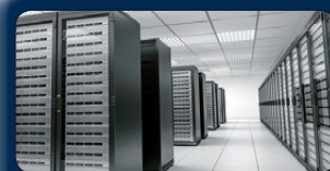
UPS & DATA CENTER
